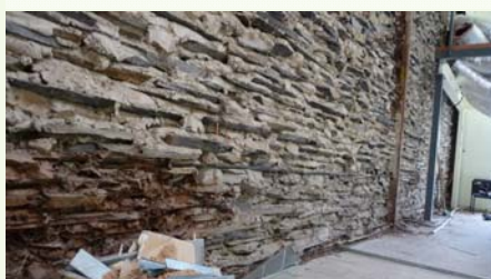
2 Remains of NE wall post termites
